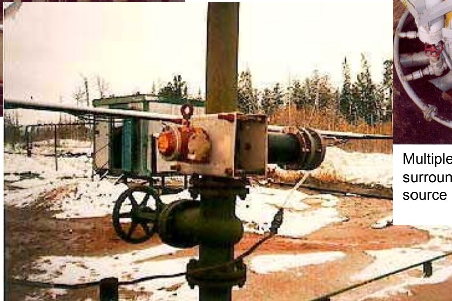
Prototype in field installation
