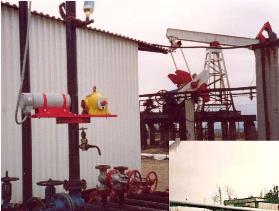
Single meter on beam-pump well
